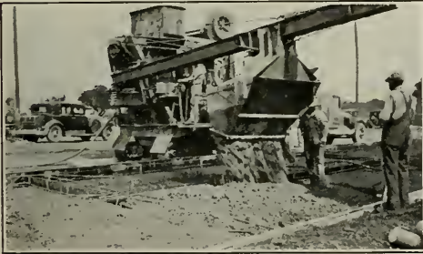
—Courtesy Pacific Portland Cement Co. Pouring concrete on Bayshore Highway, between Redwood City and Palo Alto, at 3 P. M., April 9, 1932. Basich Bros. general contractors. Golden Gate 24-hour cement used.
